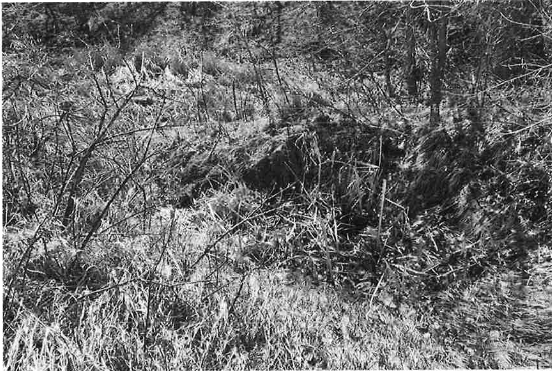
Overgrown discharge channel below 6" pvc seepage drain.
